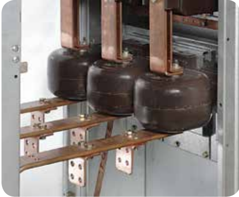
LPCT in cubicle
