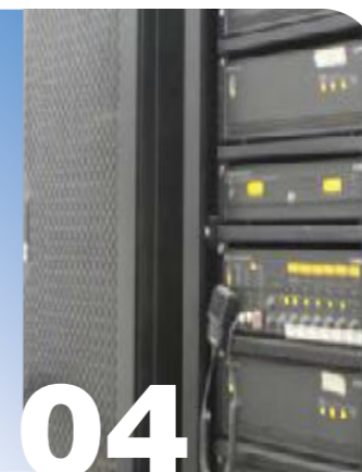
TỦ RACK Rack Cabinet
